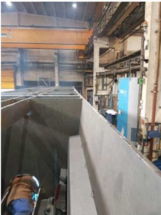
Figure 4: Clean air around the filtration tower – on the left side rising welding fumes are discernible
