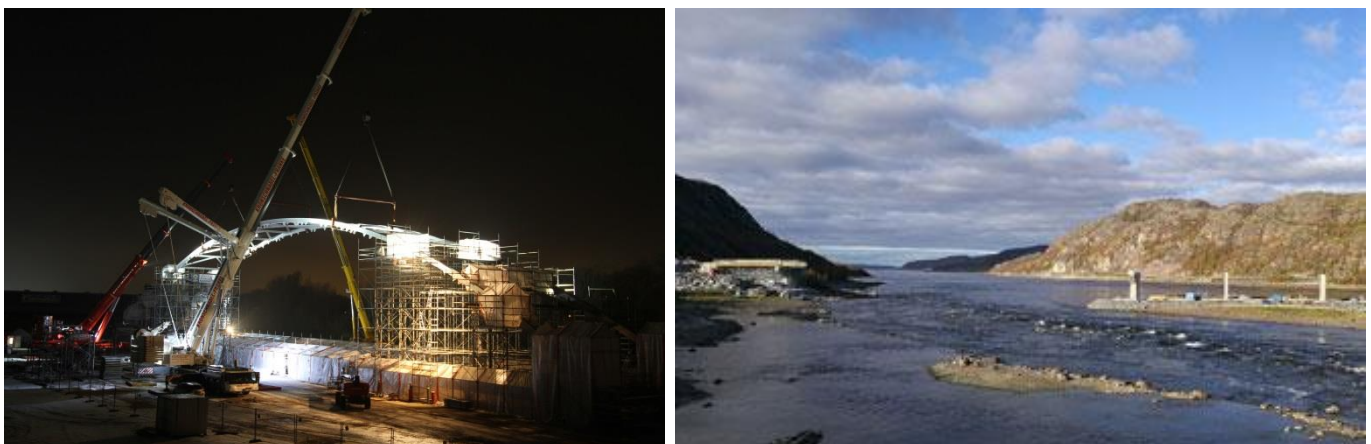
Figure 1: Main part of the arch bridge for a traffic project at the North Cape – to fill a gap of 120 meters
